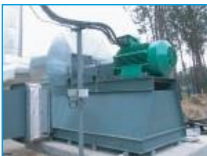
Acoustic insulation at the fan casing.
